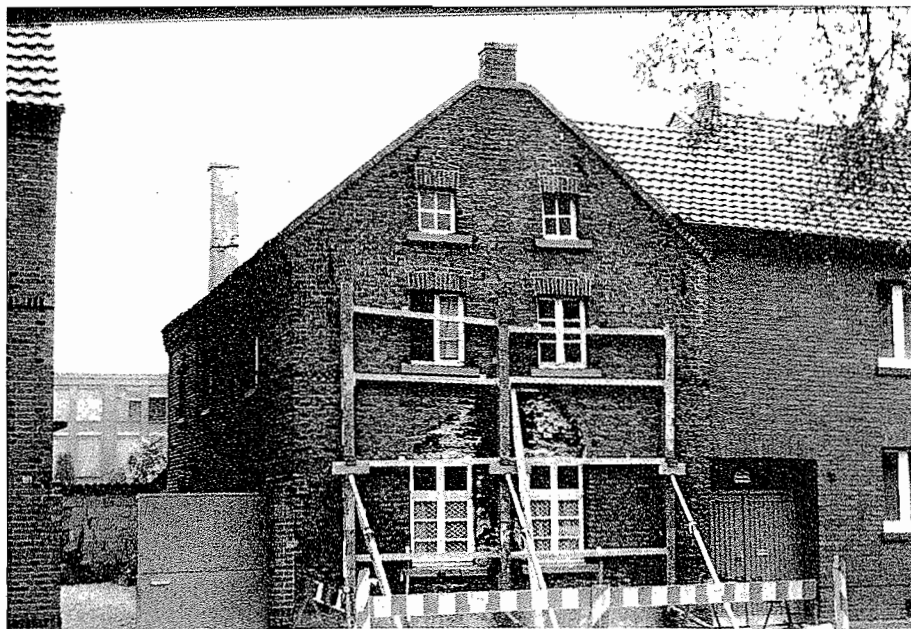
Out-of-plane failure of unrestrained wall panel in older masonry building in Heinsburg
