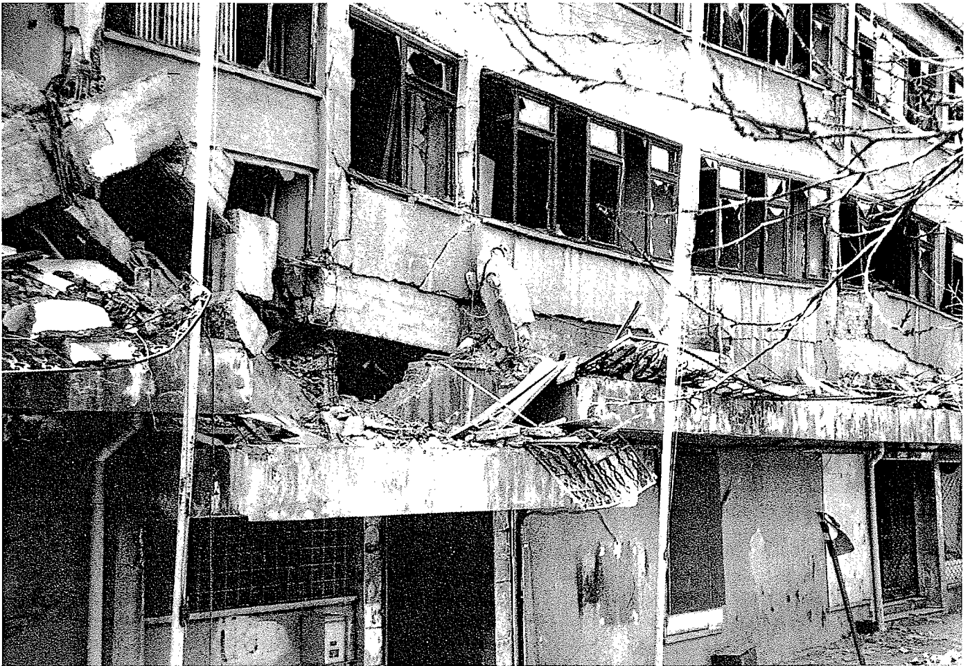
Above: Complete collapse of a storey in a reinforced concrete frame building. The upper and ground floors remain standing.
