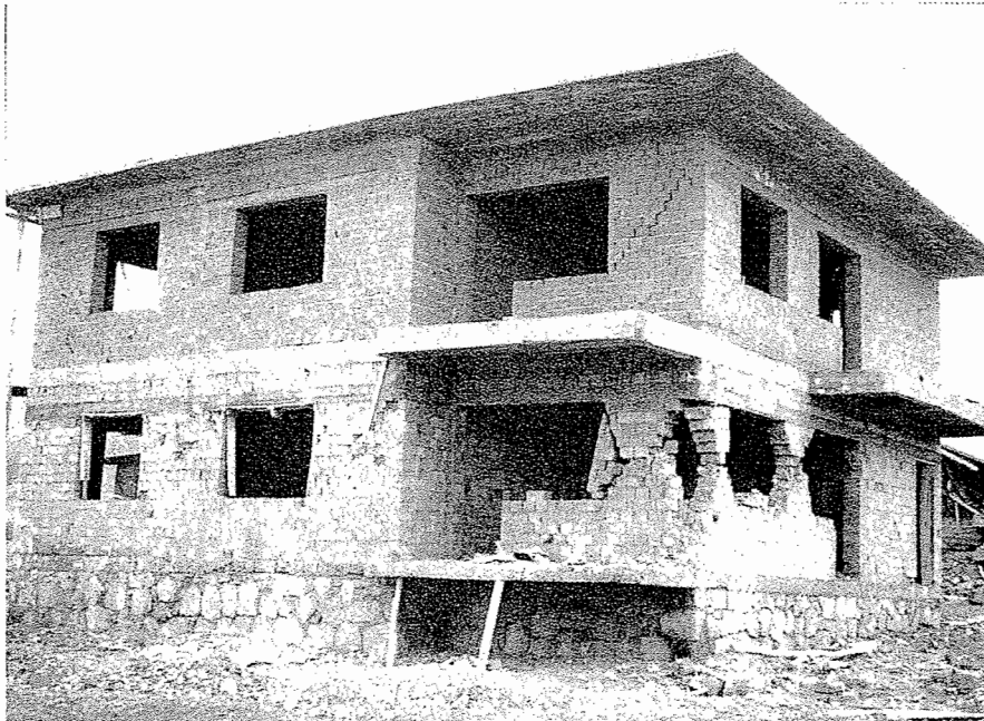
Unreinforced masonry building with reinforced concrete ring beam and floor slabs. Corner failure at ground floor level. The ring beam acts to limit scope of failure thereby protecting occupants.
