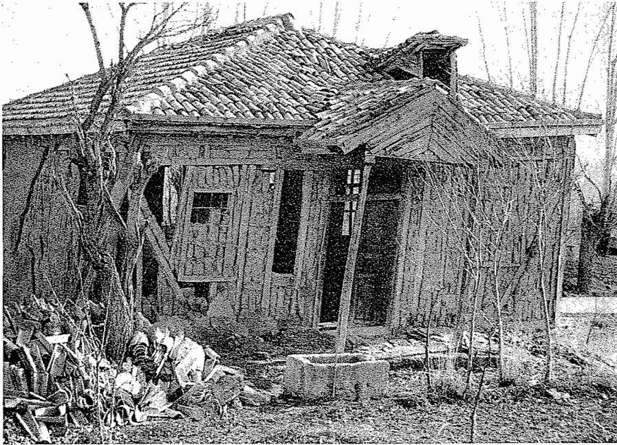
Traditional Turkish house, "Himis". It consists of timber frame with adobe infill. Most of them in the epicentral region were clearly shattered but still standing. Very little loss of life in such buildings but unfortunately timber is scarce at present in Turkey.
