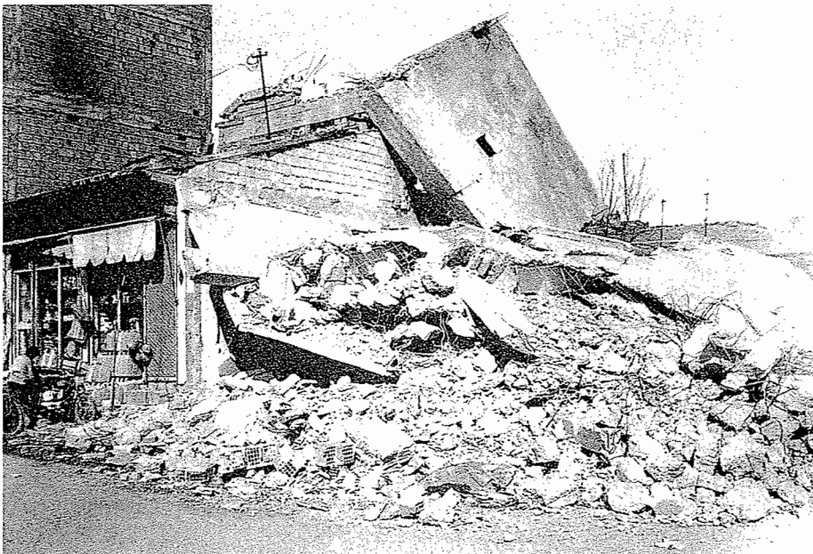
Complete collapse of a reinforced concrete frame building. Form of failure promotes high lethality potential.
