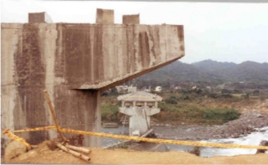
Figure 5 Effect of fault displacement on bridge – (Chi Chi Earthquake)
