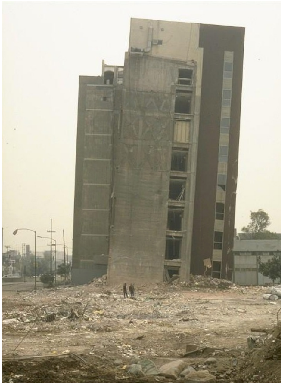
Figure 4 Failure of floating piled foundation (Mexico City)
