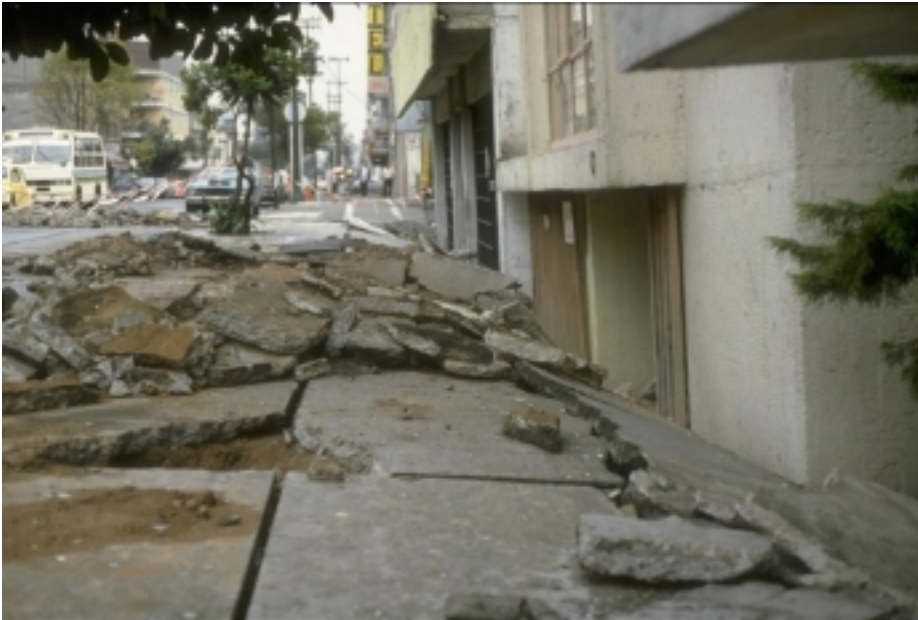
Figure 2 Bearing capacity failure (Mexico City)
