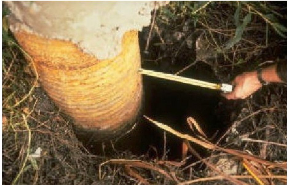
Figure 3 Gapping around piles
