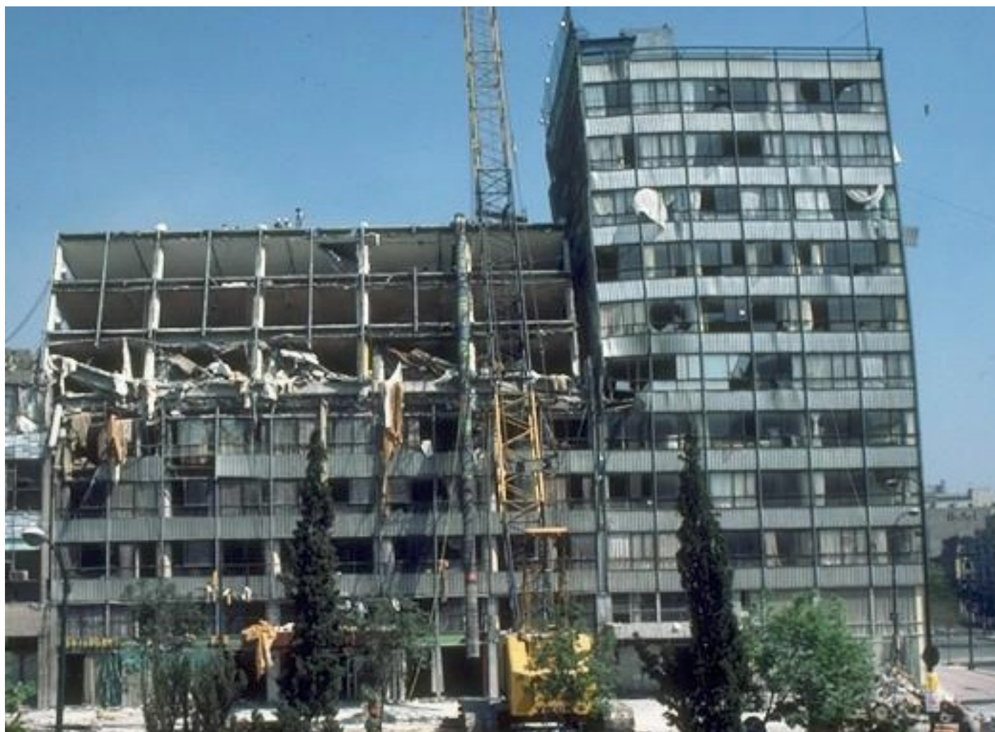
Figure 1 Mid-storey collapse due to pounding (Mexico City)
