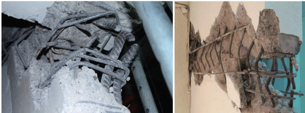
Figure 1. Low-cycle fatigue failure due to rupture of the main bars at the end of RC walls, Chile (Naeim, et al., 2011), (Youssef, et al., 2011).
