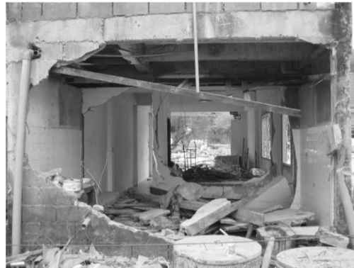
Figure 1. Punching failure of infill wall (Ruangrassamee et al. 2006).
