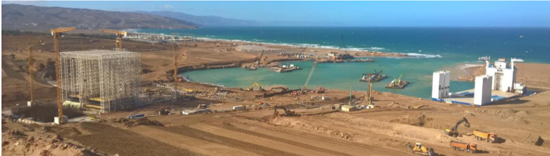
Figure 1. The Port of Nador project site during the initial phase of the project, looking north with the Mediterranean Sea in the background.
