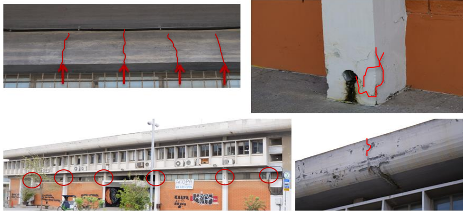
Figure 3. (a) Crack locations in beams, (b) Column base with cast-in drainage pipe, (c) Short columns due to infill brick walls, and (d) Deterioration of concrete.
