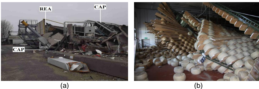
Figure 4. Examples of consequences after the 2012 Emilia earthquake (a) REA and CAP (b) PRO (source: Agenzia regionale per la ricostruzione – Sisma 2012).
