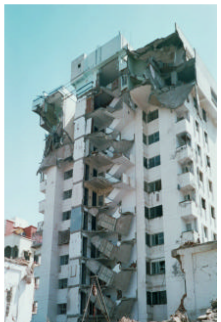
Figure 4: Collapse of the Mansi complex in Ahmedabad: a complete block identical to the one seen in the picture has collapsed
