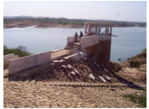
Figure 3: Failure of the appurtenant structures of Rudra Matha Dam
