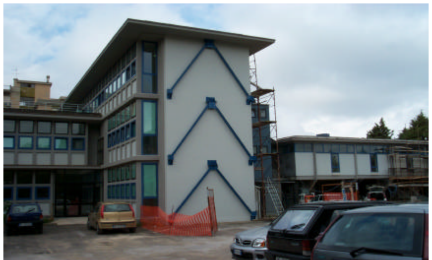
Fig.2: The damping device used to rehabilitate a school building in Italy
