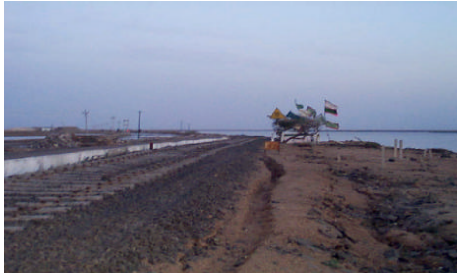
Figure 1: Lateral spreading next to the track at Navalakhi port
