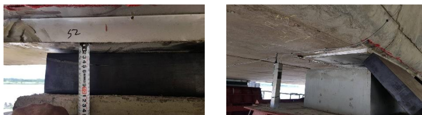
Figure 10 The unanchored bearing of NC20a
