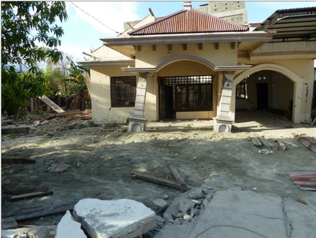
Figure 6. Damage to a one-storey building in Lasoso due to differential settlement induced by liquefaction. Sandy ejecta in garden.
