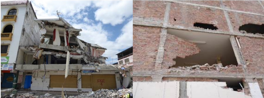
Figures 3 and 4. Collapsed building showing failure of frame, and masonry failure out-of-plane.
