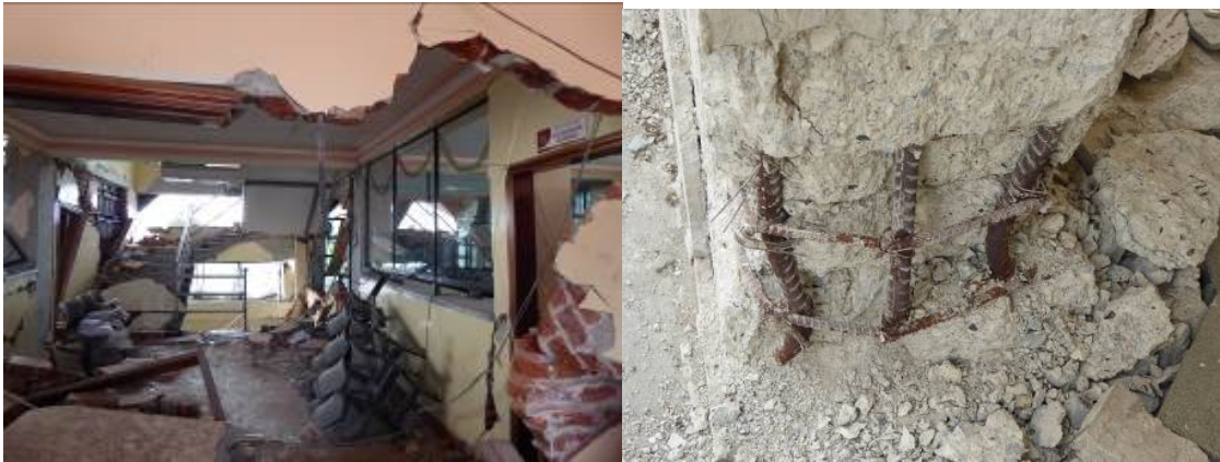
Figures 13 and 14. Inadequate securing of non-structural elements and poor quality concrete.
