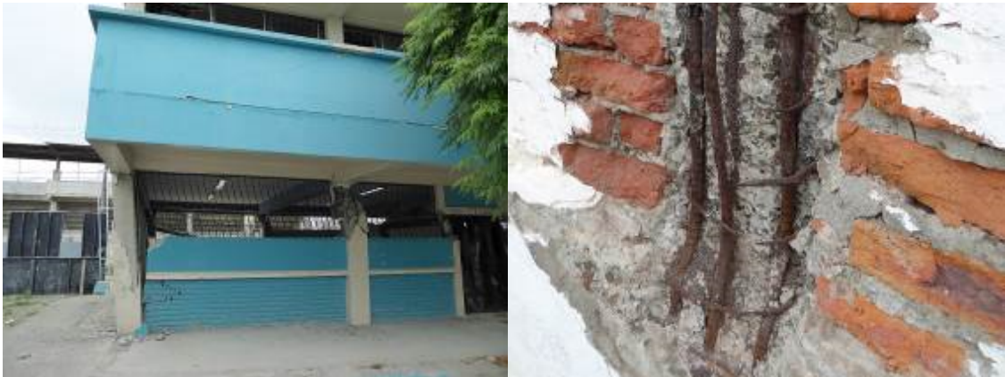
Figures 9 and 10. Short column failure and insufficient cover to rebar.
