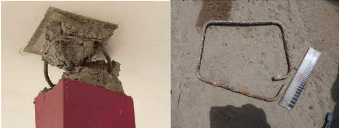
Figures 5 and 6. Inadequate design and detailing for shear –link spacing and detailing.
