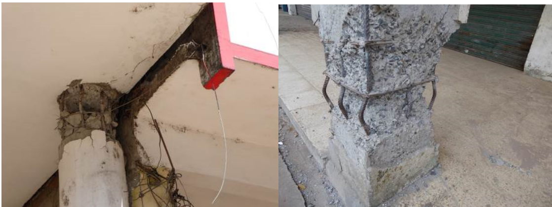
Figures 11 and 12. Pounding of a column head by a slab of an adjacent building, and inadequate design of plastic hinges.
