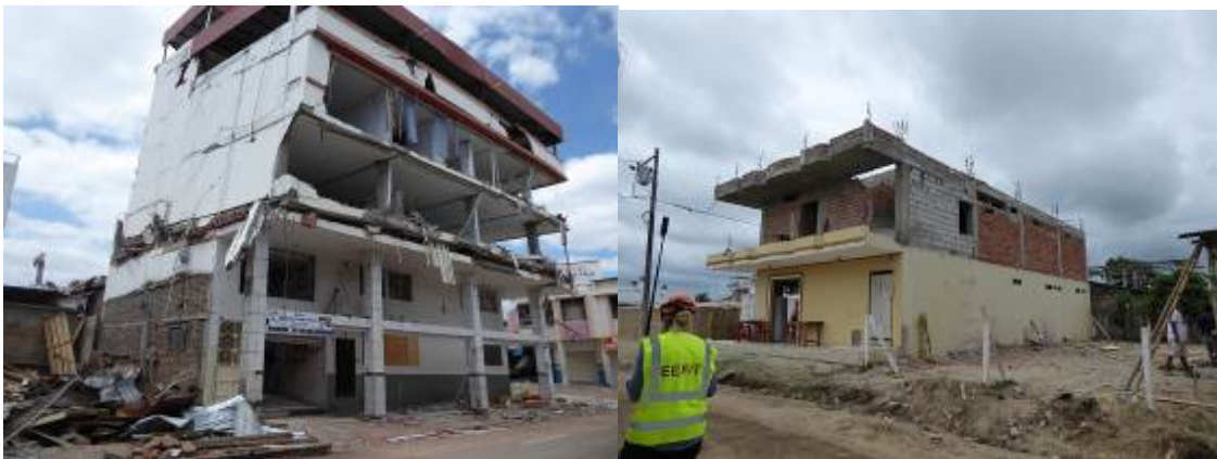
Figures 7 and 8. Weak/soft storey failure, and exposed reinforcement with possible inadequate lap lengths for future construction.
