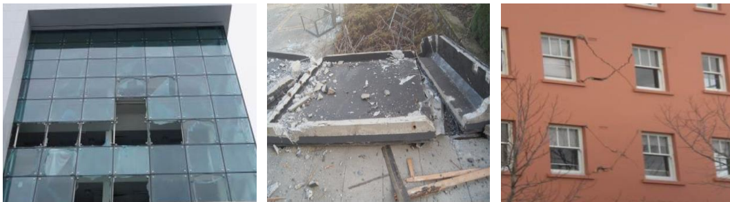
Figure 1. Examples of damage to curtain walls (left), precast concrete cladding systems (centre) and masonry infill walls (right) from Baird et al. (2011).
